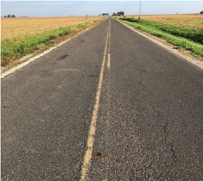
Original Narrow, Distressed Pavement
