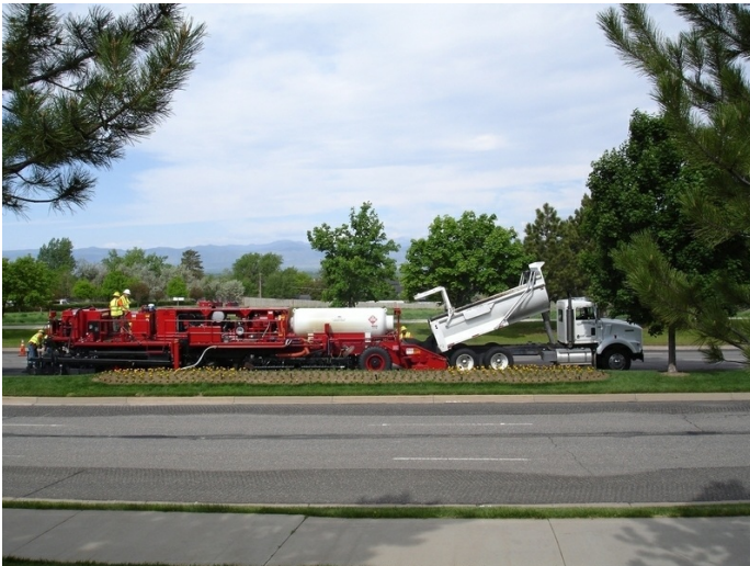
Cutler Repaving's single pass recycling process completes the recycling and resurfacing simultaneously, thereby minimizing delay and inconvenience to the traveling public.
